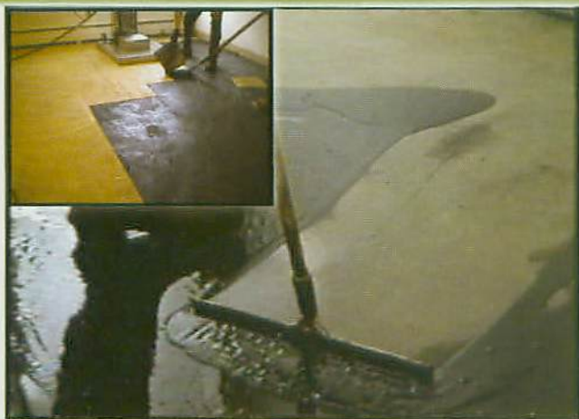
Remove asbestos mastic!
